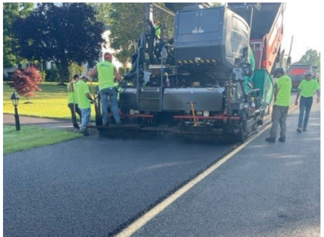
Ultra-thin overlay process being applied to Mininger Road. Double Seal Coat followed by Polymer Modified Fog Seal process
