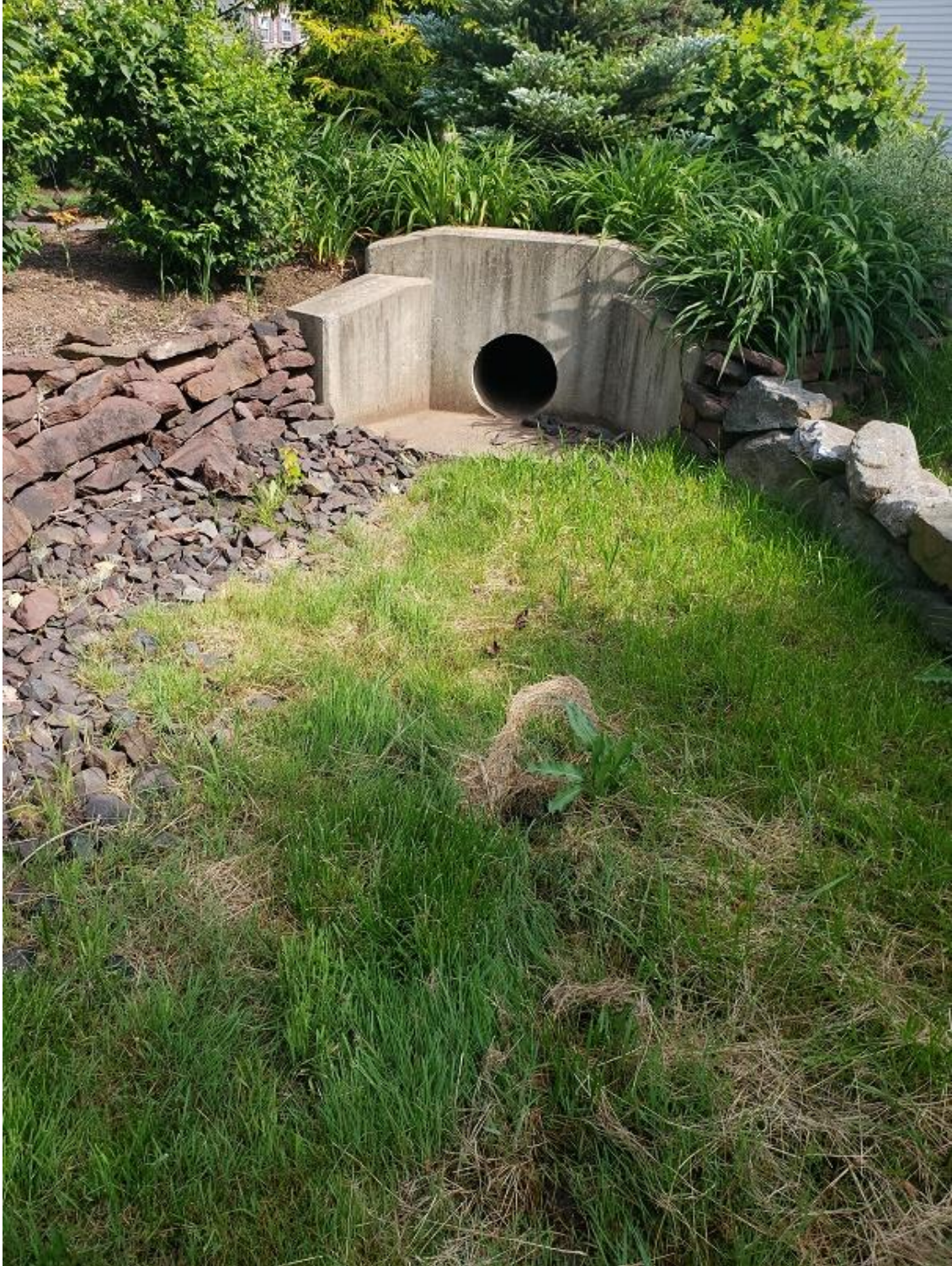
Endwall located on 334 Elmwood Lane. I believe the beginning of the Indian Creek tributary begins in this area. The stormwater from Telford Pike makes its way to this endwall.
