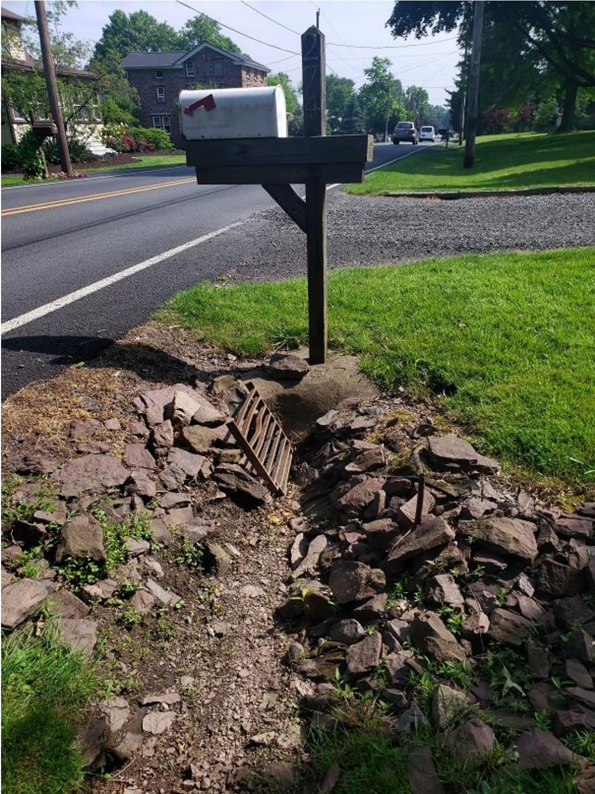
End of ditch along Telford Pike. The ditch ends in front of 274 Telford Pike. Under the grate is the beginning of the cross pipe that take the stormwater under Telford Pike and under the property of 261/263 Telford Pike.
