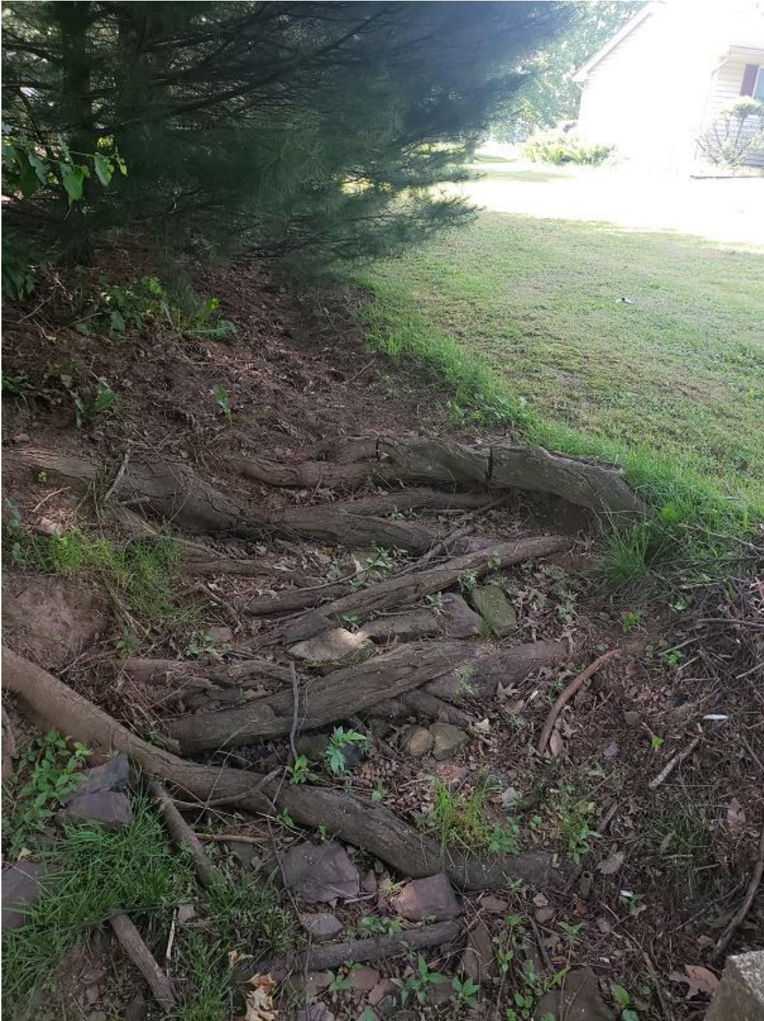
Eroded Channel on the property of 284 Telford Pike. This channel discharges along Telford Pike and seems to be the origin of the ditch along Telford Pike
